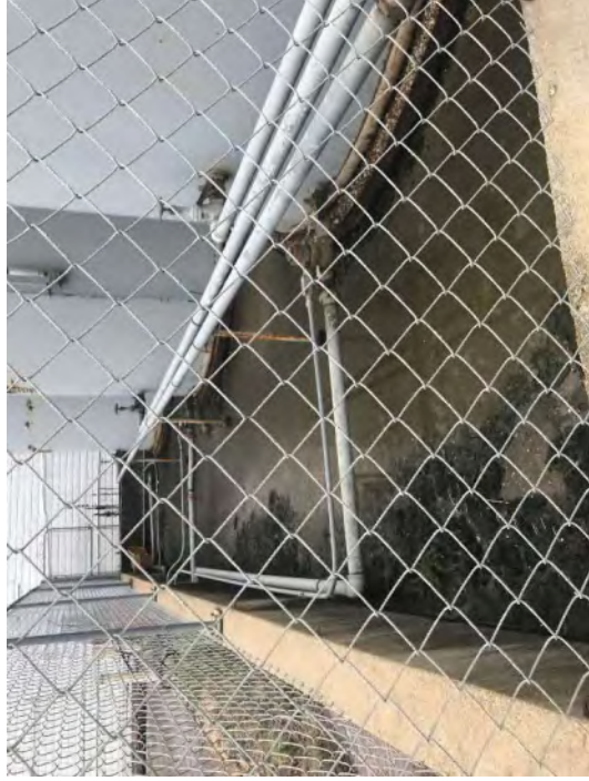
Photo #7 View of the AST containment area and associated piping.
