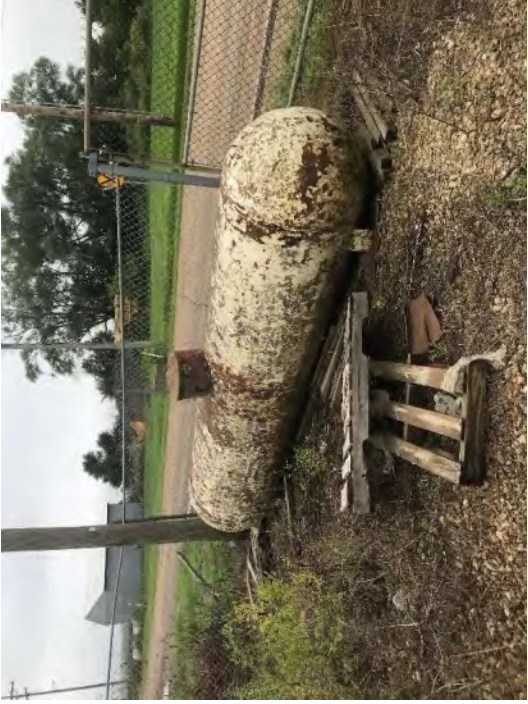
Photo #13 View of a propane tank located in the western fenced area located on the west side of the onsite building.
