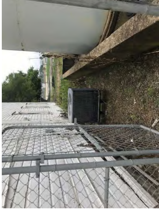
Photo #8 View of an air conditioning unit located between the building and the AST farm.
