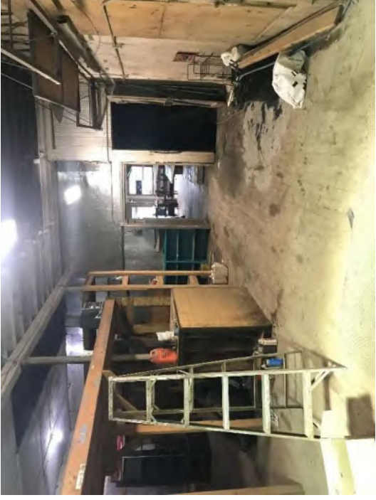
Photo #26 View of the southern portion of the first floor of the Midland Feed Store building.
