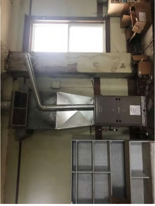
Photo #30 View of the furnace located on the second floor of the Midland Feed Store building.
