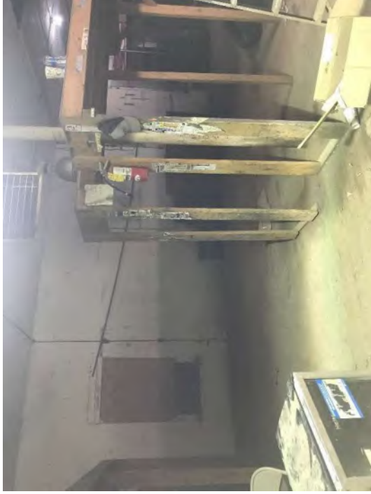
Photo #27 View of the southern portion of the first floor of the Midland Feed Store building.
