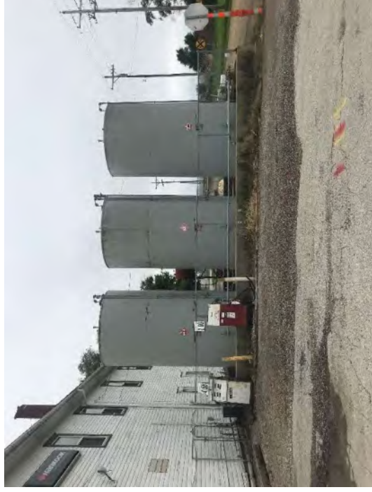
Photo #4 View of the AST tank farm and two dispensers located on the west side of the onsite building.
