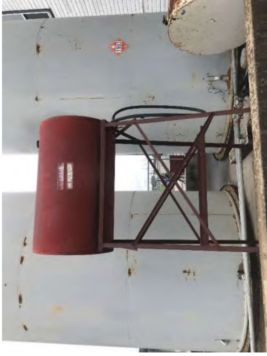
Photo #10 View of an unmarked AST located in the AST containment area.
