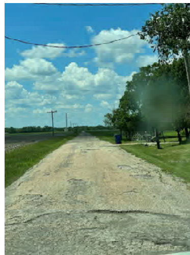
N 2000 Rd: Broken Pavement/Potholes near driveway of home
