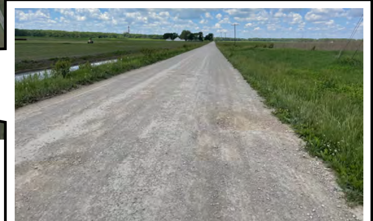
N 1900 Rd: Series of potholes west of E 1400 Rd
