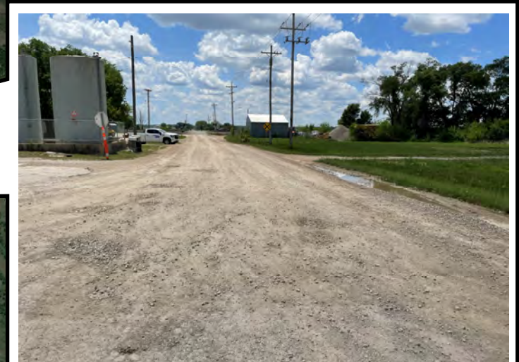
Series of potholes and standing water b/w RR X-ing and US-59
