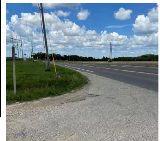
E 1400 Rd: Broken pavement on approach to US-59
