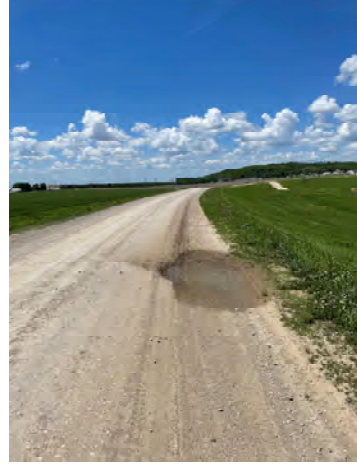
N 2000 Rd: Series of potholes, rutting, and standing water east of E 1400 Rd
