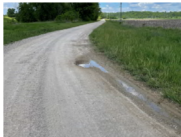
E 1250 Rd: Potholes & rut north of N 2000 Rd
