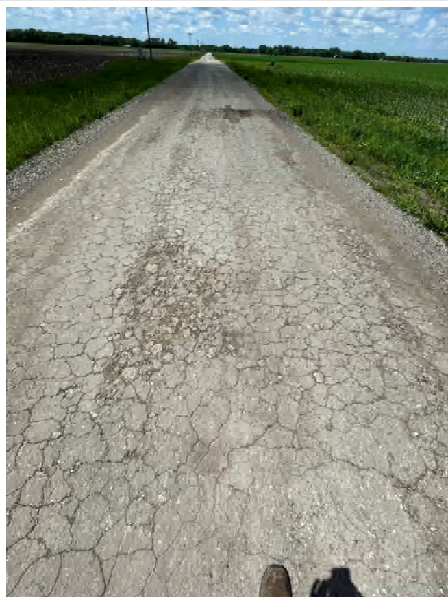
N 2000 Rd: Broken Pavement/ Potholes west of E 1400 Rd
