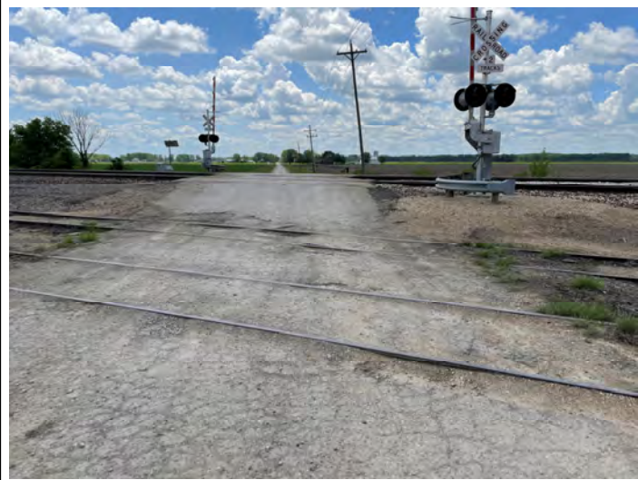
E 1400 Rd: Broken Pavement/Potholes at RR X-ing
