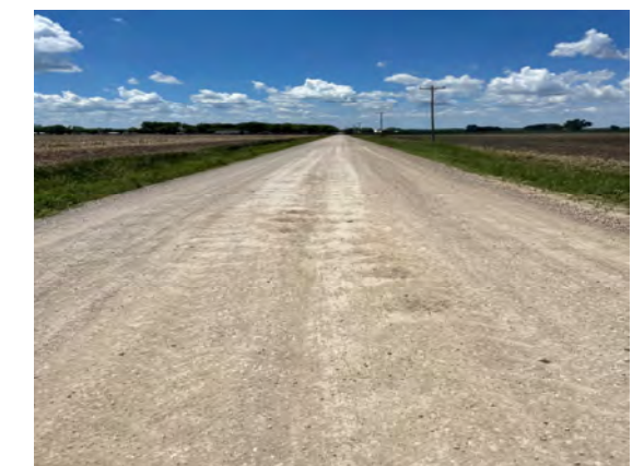
N 1900 Rd: Series of potholes west of E 1500 Rd
