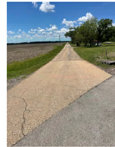
N 2000 Rd: Cracked pavement on W of US-59
