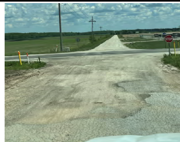
N 1900 Rd: Broken Pavement/ Potholes west of US-59
