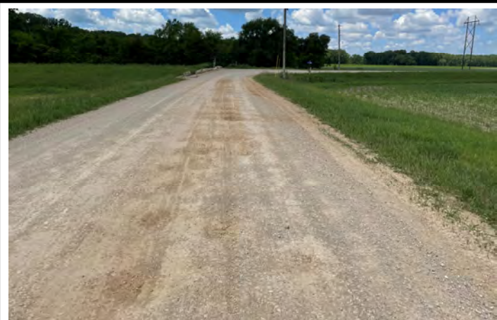
N 1900 Rd: Series of ruts & potholes east of E 1300 Rd
